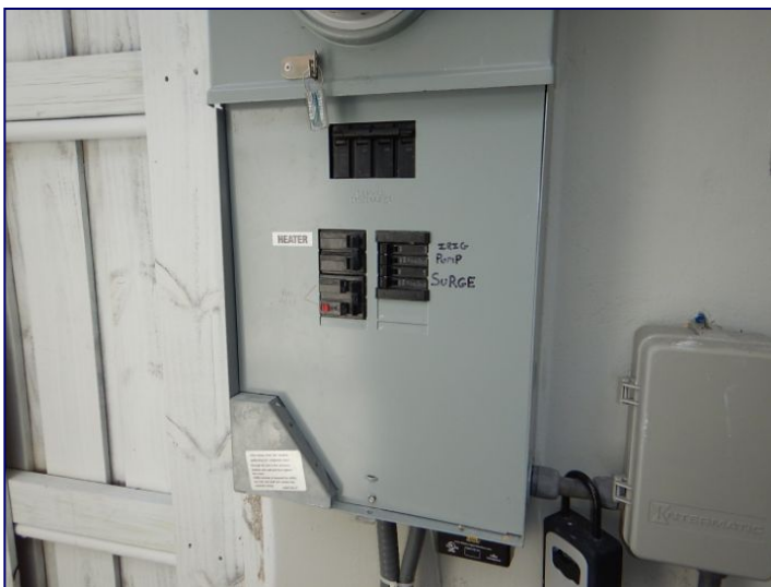
EXTERIOR MAIN DISCONNECT:
