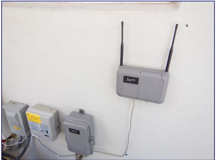
The pool heater controls are locked and the heater appears to be controlled by an Aqualink type remote control system. Heater could not be evaluated for operations. Have seller demonstrate operations prior to closing.
