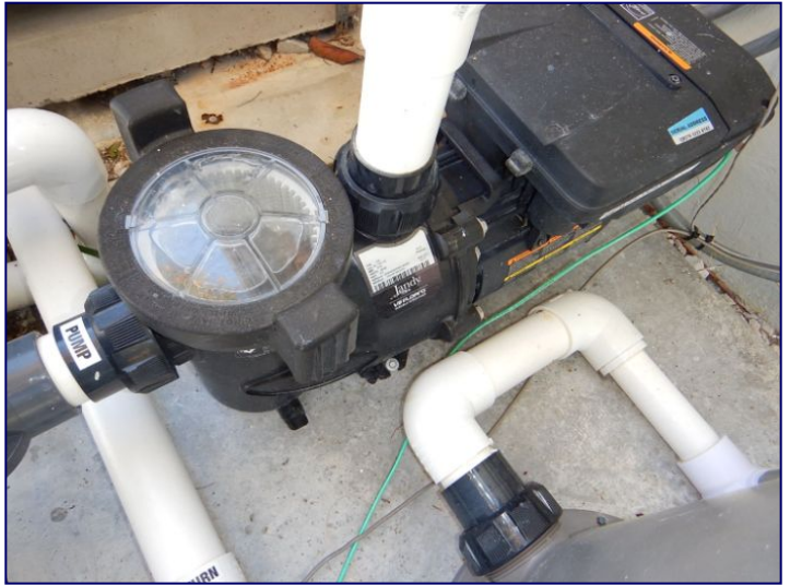
Pool motor appears to be properly grounded at the time of inspection.
