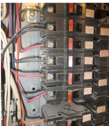
A Federal Pacific Electrical panel
