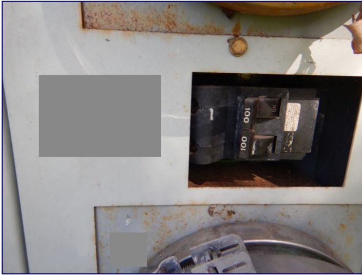
Main amperage coming into the home.
